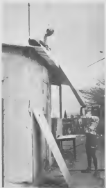
Rey Barro, not only works at the top of the organization, but also on top of a roof. Rey Barro, no solamente ariba den e organizacion, sino ariba un dak pa traha tambe.
